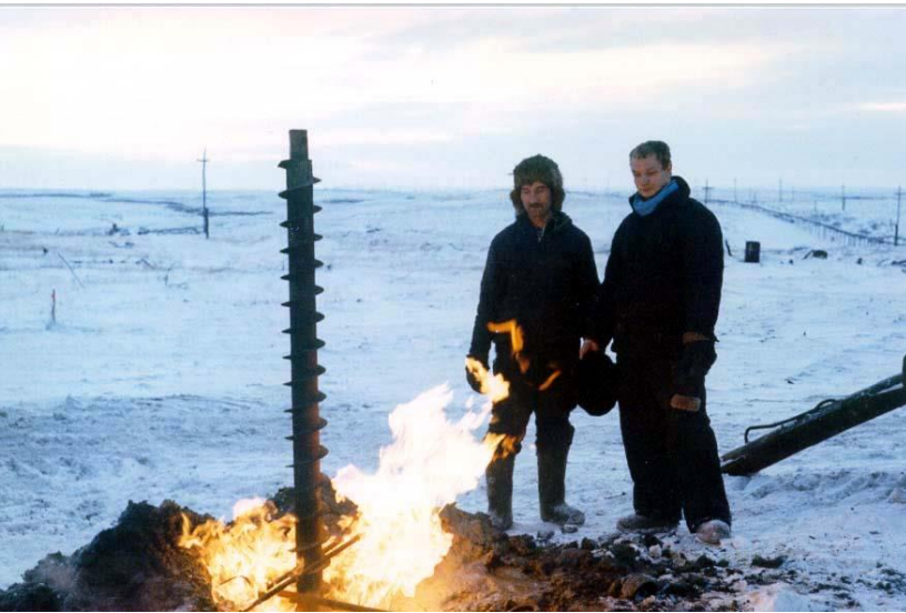
Fire when drilling monitoring well
