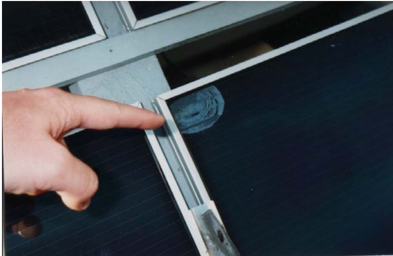
FIGURE 6. WATER INTRUSION RELATED DELAMINATION IN A SHENZHEN TOPRAY A-SI SOLAR MODULE. PHOTO: ARNE JACOBSON.
